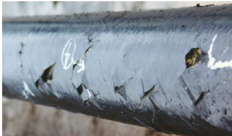
Figure 10-1: Pipe that exhibits many coating holidays. Pipe was coated in the late 60's and dug up in 1996. 2
