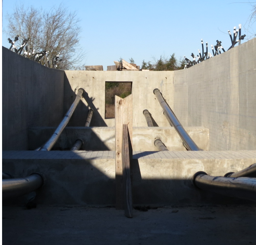
Figure 6-2. An image of the inside of the mock bridge built at Texas A&M.
